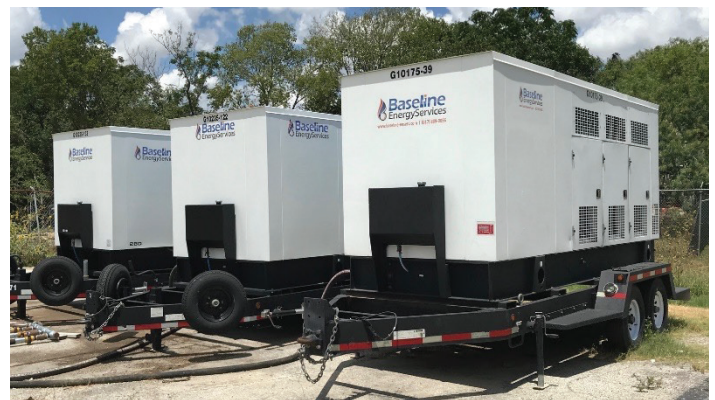
Baseline™ 3 x 175 kW natural gas generators (525 kW total available power).
