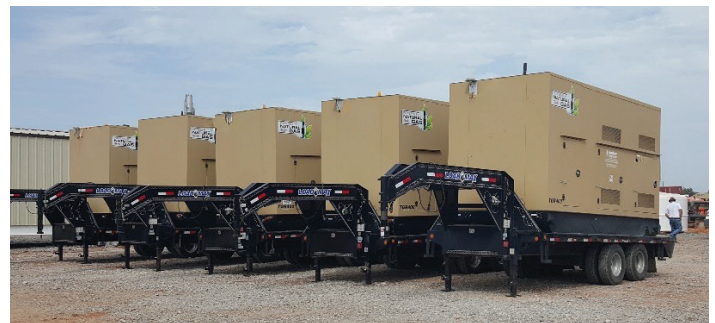
Five (5) of an eventual ten (10) x 350 kW Baseline™ mobile natural gas generators setup to provide power to an Oklahoma gas and electric utility.
