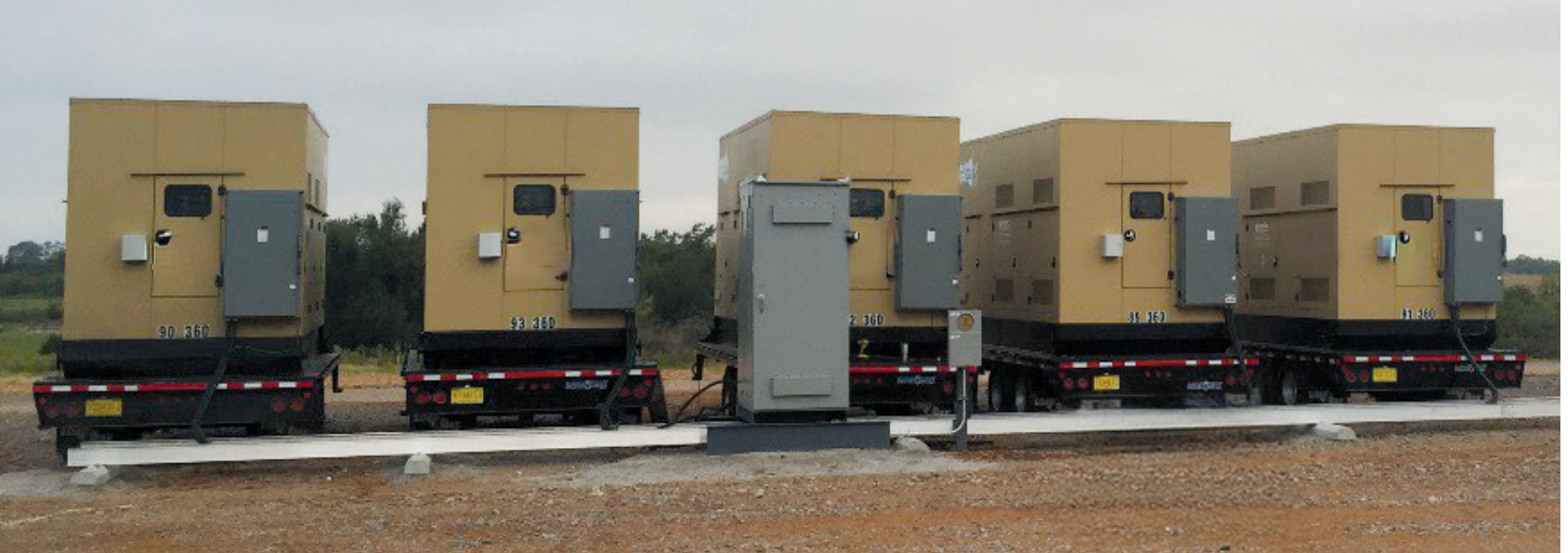
Five (5) of an eventual ten (10) (3.5 MW) Baseline mobile natural gas generators system that is providing reliable electric power to an Oklahoma gas and electric utility.
